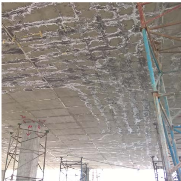
Fig. 9 Crack distribution (raw image)
